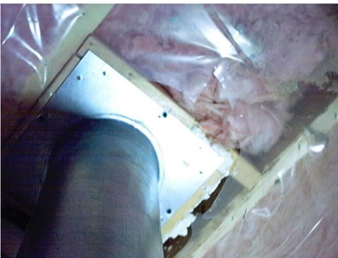
Chimney chases are often leakage areas.
