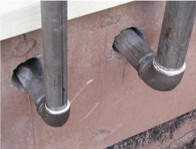
Oil filler pipes should be sealed from the outside and foamed from the inside.
